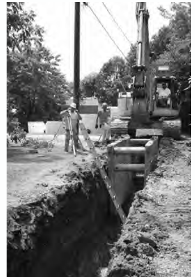
Employees of Field's Excavating of Kitts Hill, Ohio work to install a sewer line in an alley way as part of the Miami County Brandt Sewer Project.
