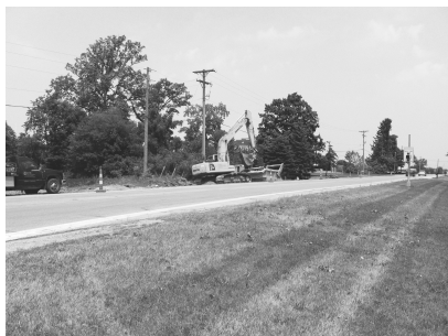
Crews from Tom’s Construction work to install sanitary sewer lines on SR201 just north of Dayton-Brandt Road.
